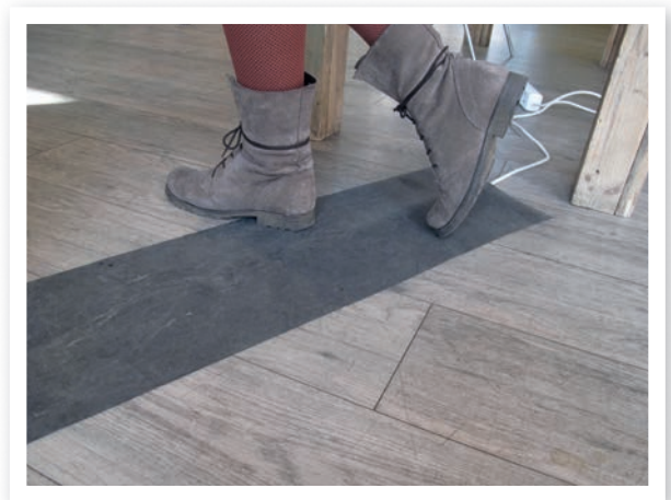
Safe: extension cords covered with rubber mats
